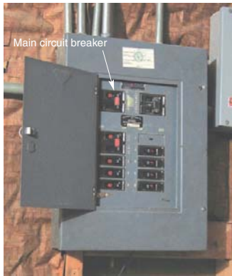
Main circuit breaker is the disconnect switch
