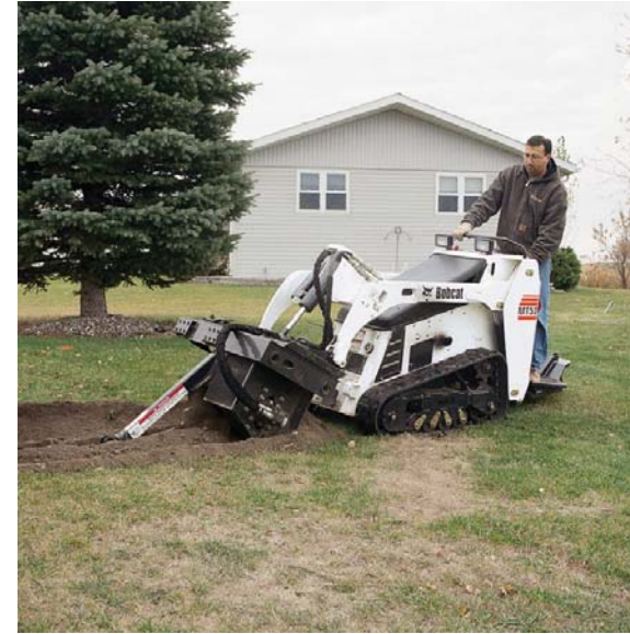
Installing underground service cable requires a trench of sufficient depth. The depth is mandated by local codes, but is usually 18" to 24". A trencher is able to dig 2' to 5' without destroying the nearby grass. (Bobcat Company)
